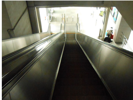
Figure 6: Escalator behind the door.
